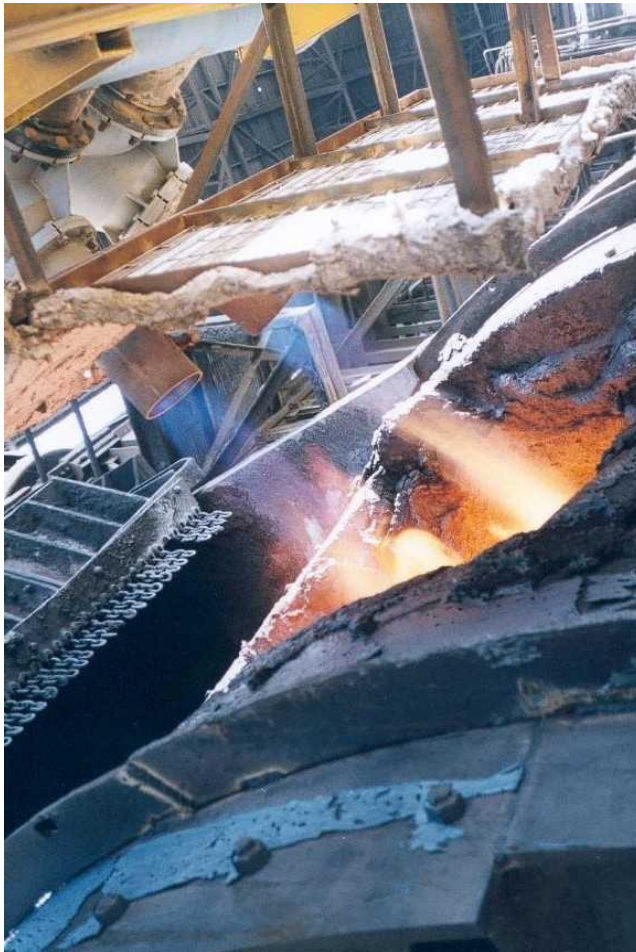
Fig. 7.1 Photo of Burners Installed in P&S Furnace
